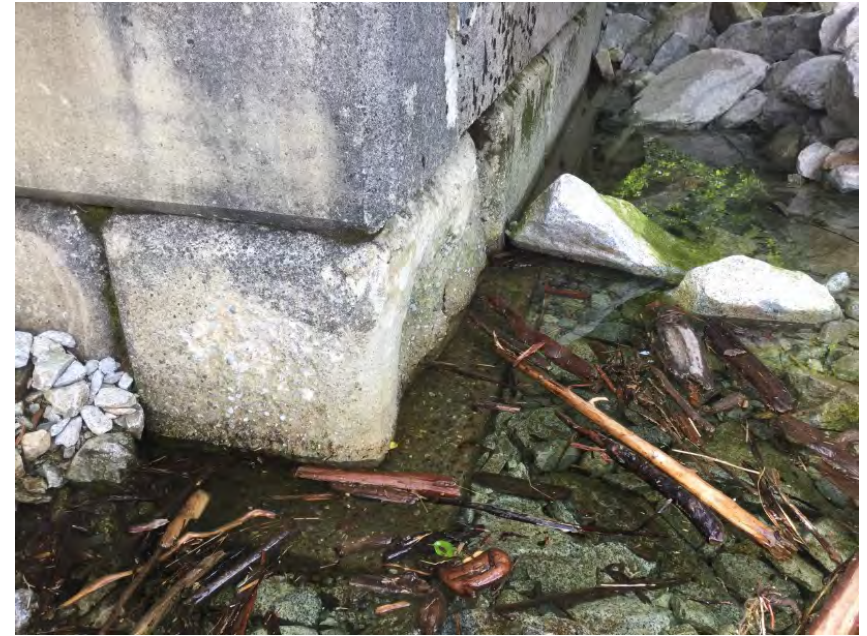
Bottom lock block at downstream right abutment in poor condition
