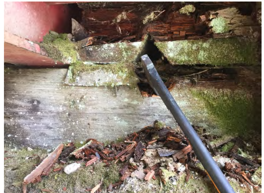
Timber sill condition
